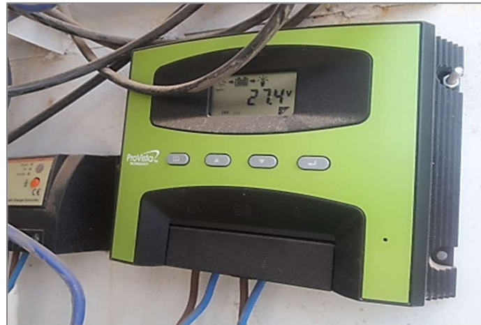
Fig. 12. A charge controller (12/24 DC).
