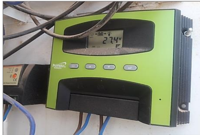
Fig. 12. A charge controller (12/24 DC).
