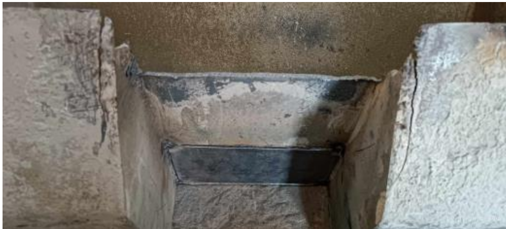
Figure (2): a bucket with cracks.
